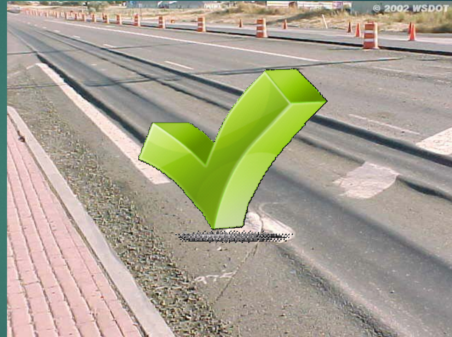
Surface Failure – Milling Required
