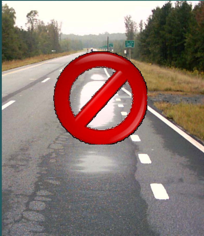
Severe Structural Failure
